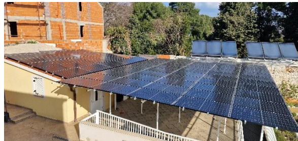
FIGURE 1: EXISTING PV SYSTEM SOLAR-1
