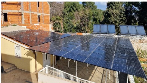
FIGURE 2: PV SYSTEM PHASE SOLAR-1
