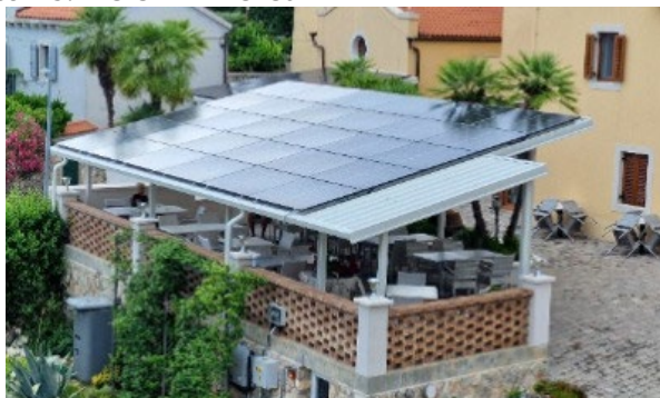
FIGURE 3: PV SYSTEM PHASE SOLAR-2
